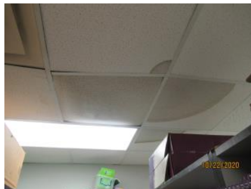
Damaged accoustical ceiling system.
