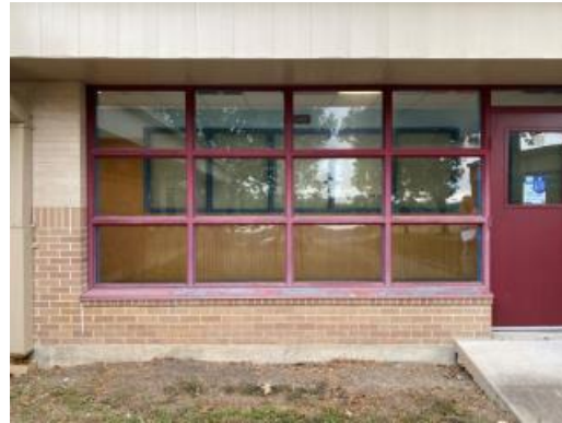
The exterior windows are in need of maintenance.
