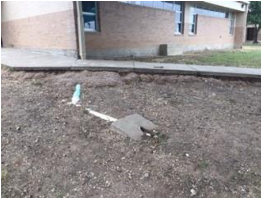
Exposed drainage pipe
