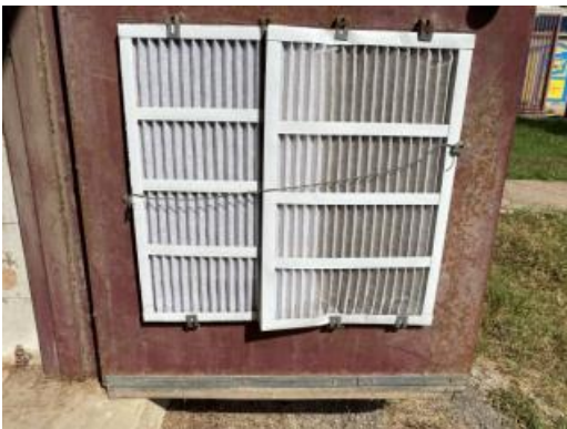
Door at the mechanical room is warped
