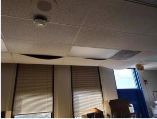
Warped/damaged acoustical ceiling tile
