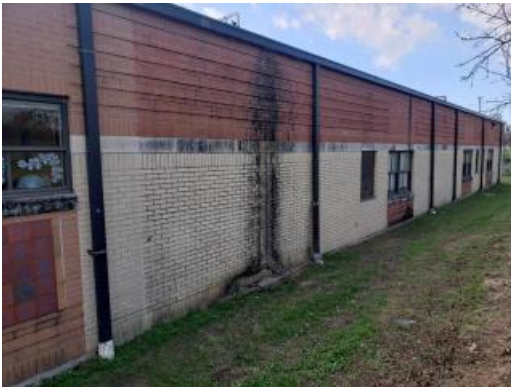
Stained brick wall
