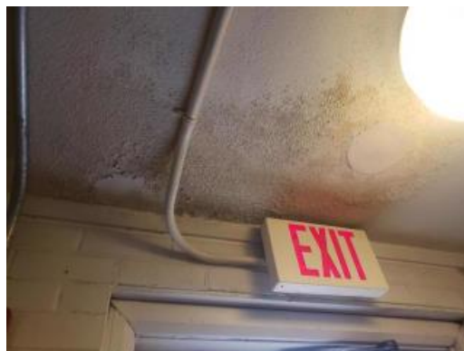
Stained plaster ceiling
