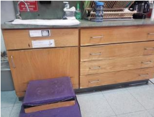
Casework finish is worn and damaged
