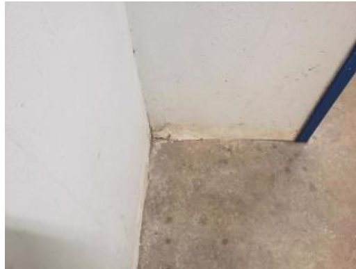
Damaged wall seal
